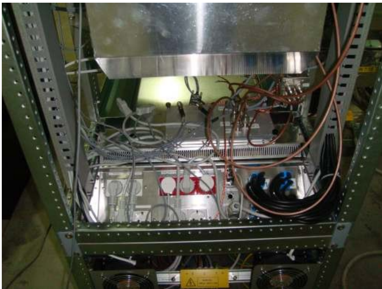
AC DISTRIBUTION AFTER TRANSFORMER
